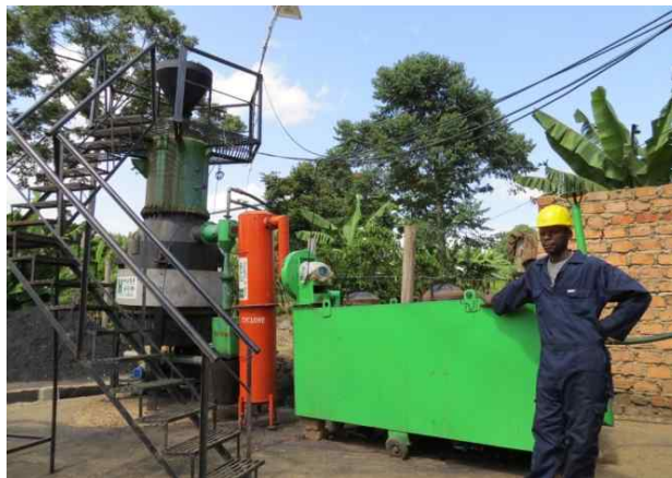
Figure 8 Biomass gasification power plant in a microgrid operated by Pamoja Energy Ltd
