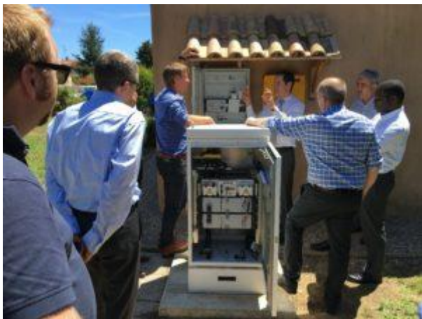
Inspection of one of the households with PV on roofs, inverter wall and battery pack placed one meter from the house wall
