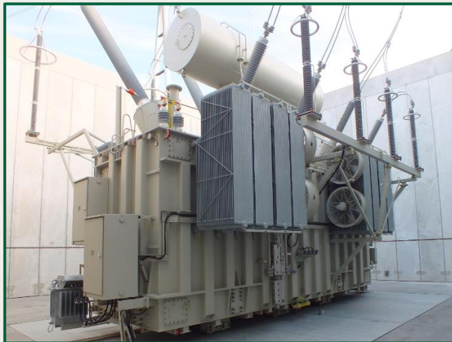
200MVA Transformer (420/66 kV)
